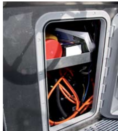
Twin batteries are tucked up amidships as part of the centre-console.
